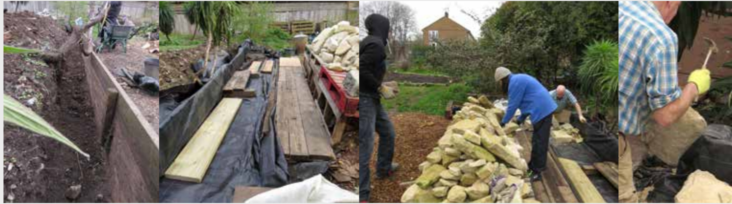
There has been a lot of work out here this year. The ground is cleared of bindweed ready to build the dry-stone wall, left; the work-space set up with re-used stone; John Holt starts work with students and volunteers.
